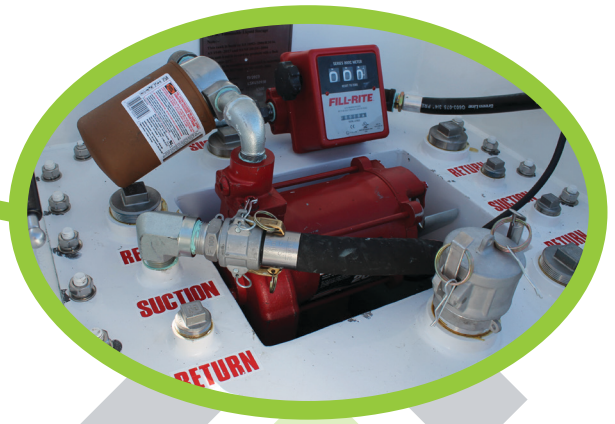
Tank Manway Recessed Spill Box Area *20 GPM Pump Shown
